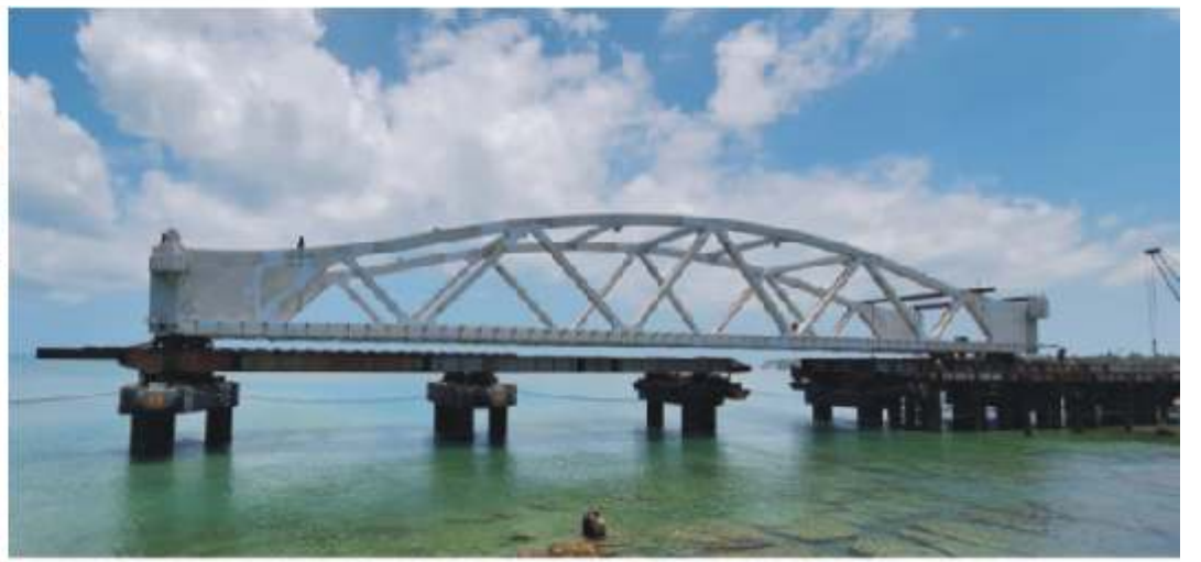
Vertical lift span portion of the Pamban Bridge being moved to its location in a phased manner
