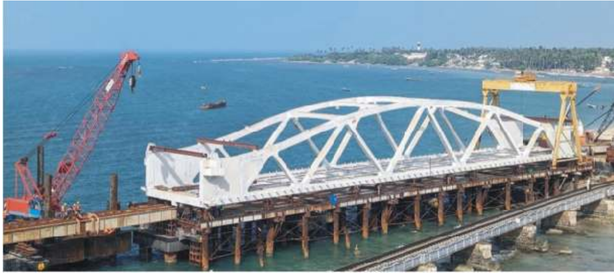
Vertical lift span portion of the Pamban Bridge being moved to its location in a phased manner
