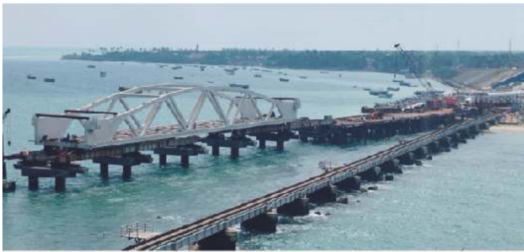
Vertical lift span portion of the Pamban Bridge being moved to its location in a phased manner
