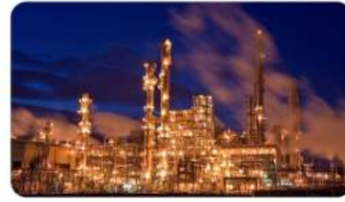
Power Plant Jam Nagar - Reliance
